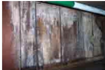
Heavy mold growth on wood ceiling rafters
